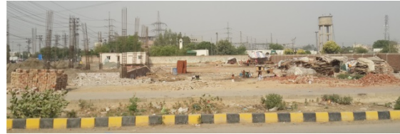
Fig. III. Commercial construction site in Johar Town right next to place where gypsy's community were living from past 11 months
